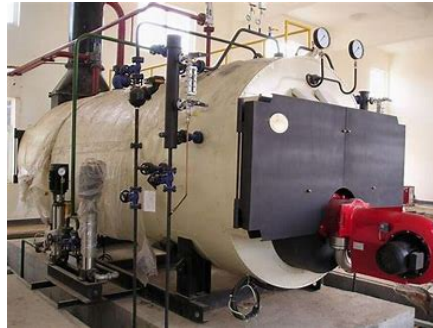
Natural gas boiler
