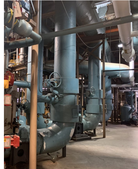
Condenser water pipes
