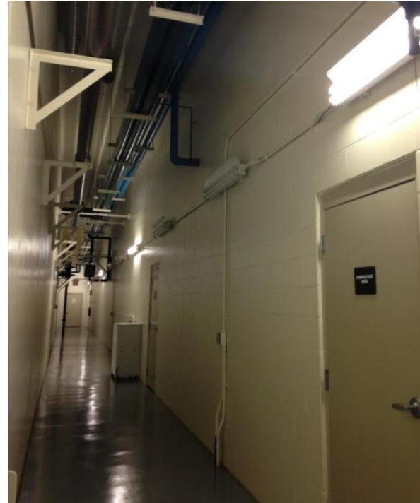
Main hall lighting
