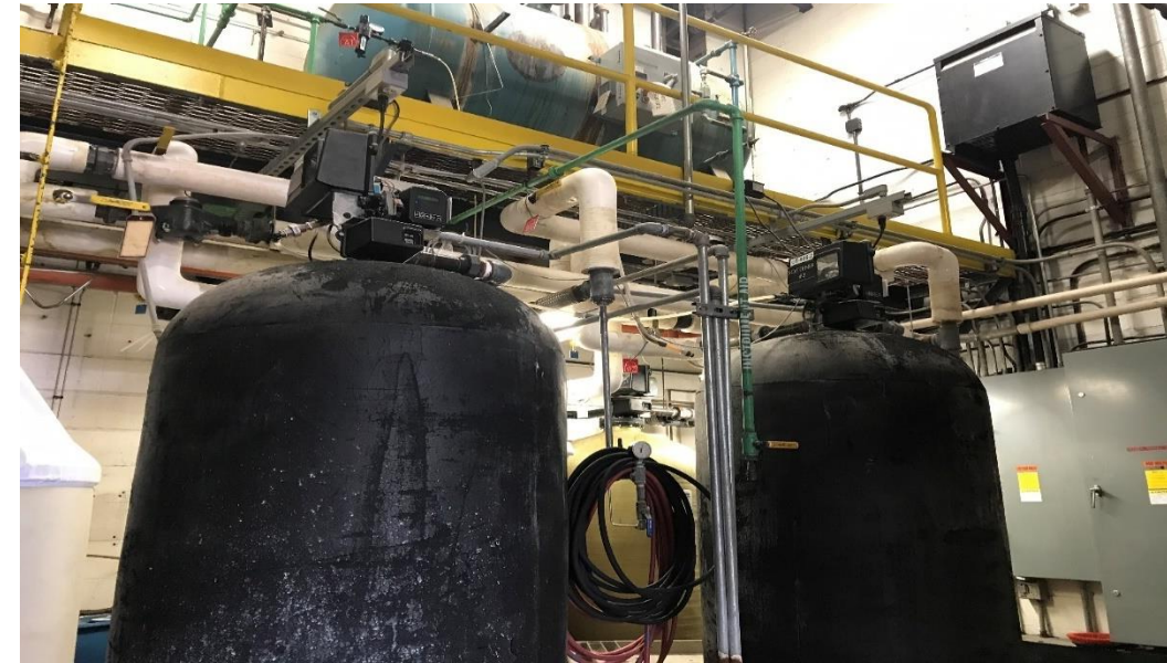
Water Softening for Boiler Water
