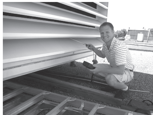
A MnTAP intern analyzed the current energy use at Nordic Ware. Here he is checking the air flow at a roof make-up air unit.
