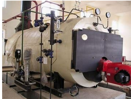
Natural gas boiler
