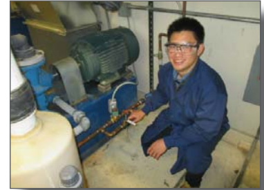
MnTAP intern, Yohanes Agustinus, looking for leaks.
